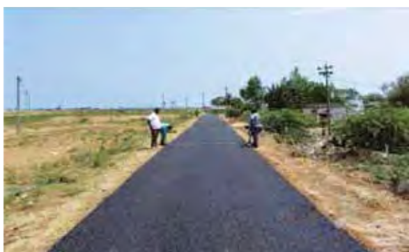
Road from Pedapattapupalem to Nandempuram of Kavali mandal in Nellore dt on 06.03.2014. MSS check (DEE present). Total length : km 2.844 (BT : 2.844KM)
